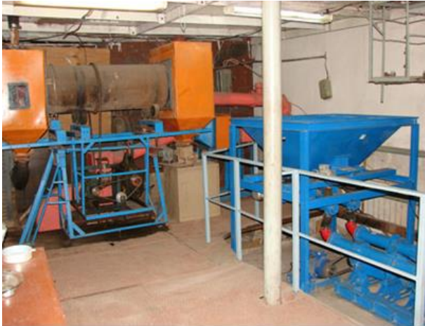
Figure 3 – General view of the pilot plant
