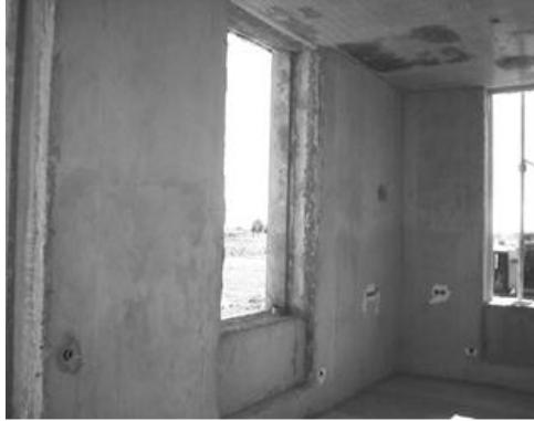
Figure 2 - Detail of the interior of a residential two-story house erected using aerated concrete wall panels
