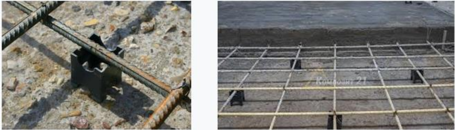
Figure 1 View and location of steel frames of the road reinforced concrete bridge protective layer
